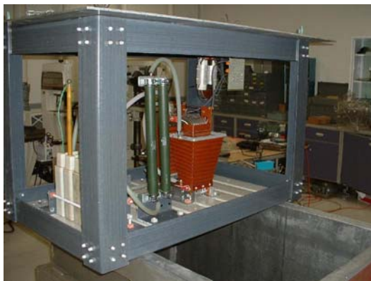
Figure 7. Photograph of the high voltage transformer (copper colored) being installed in the modulator.
